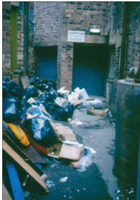
Figure 9: A blocked escape route (courtesy of the Association of British Theatre Technicians)
