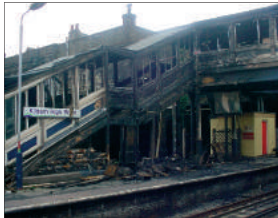
Figure 19: Fire in an air-handling unit (electrical) (courtesy of Network Rail)
