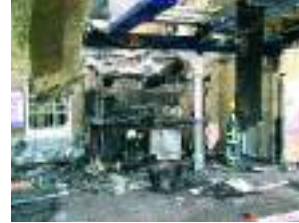
Figure 6: Fire in a retail unit on a platform (arson) (courtesy of Network Rail)
