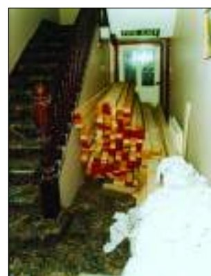
Figure 9: A blocked corridor with incorrect signage
