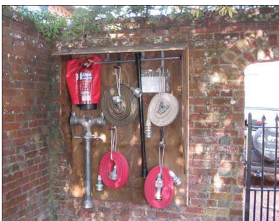
Figure 18: Provision of firefighting equipment
